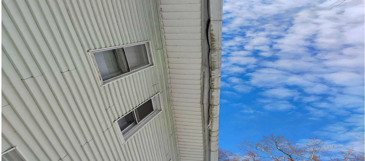
Deterioration of original cornices and eaves
