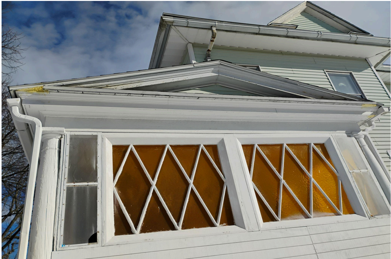
Urgent restoration: historic cornice, eaves and drainage system integration
