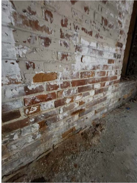
Photograph #30 – Deteriorated Interior Masonry
