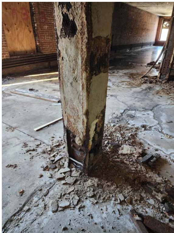
Photograph #19 – Cracked Concrete/Plaster Encasement
