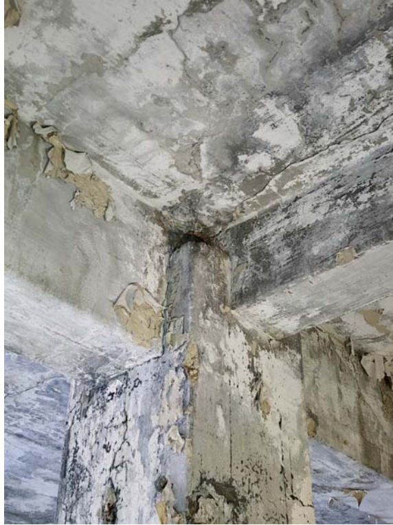
Photograph #18 – Cracked Concrete/Plaster Encasement
