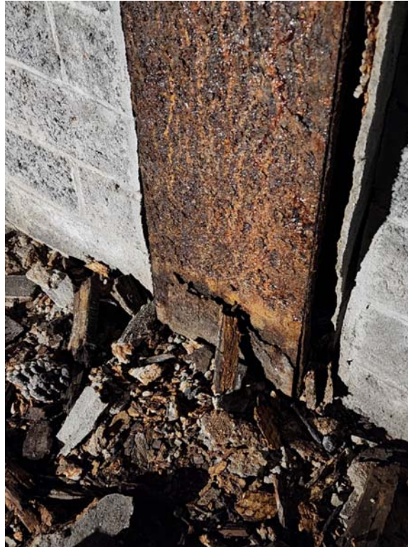
Photograph #24 – Corroded Steel Column
