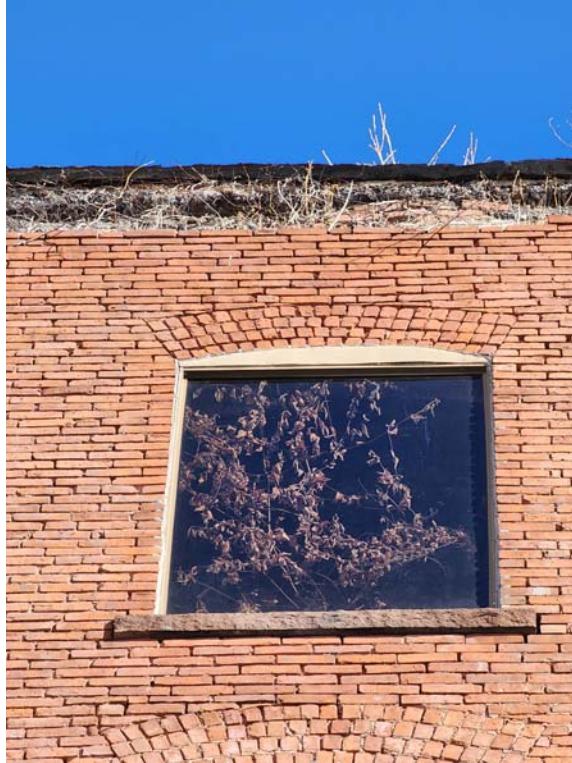
Photograph #11 – Tree Inside of Building
