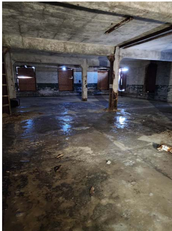
Photograph #2 – Ice on Upper Floor Level
