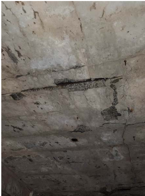
Photograph #12 – Cracked and Spalled Concrete Slab (Underside)
