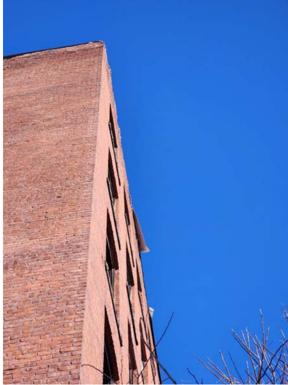
Photograph #40 – Failed Roofing/Flashing
