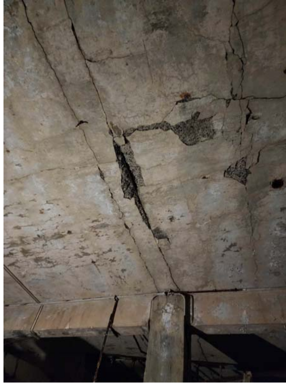
Photograph #13 – Cracked and Spalled Concrete Slab (Underside)
