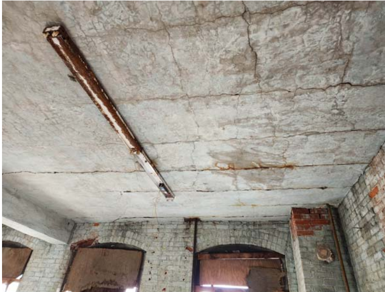
Photograph #15 – Cracked Concrete Slab (Underside)
