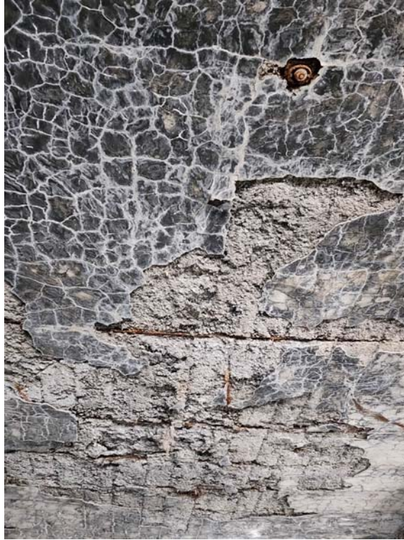
Photograph #16 – Cracked and Spalled Concrete Slab (Underside)
