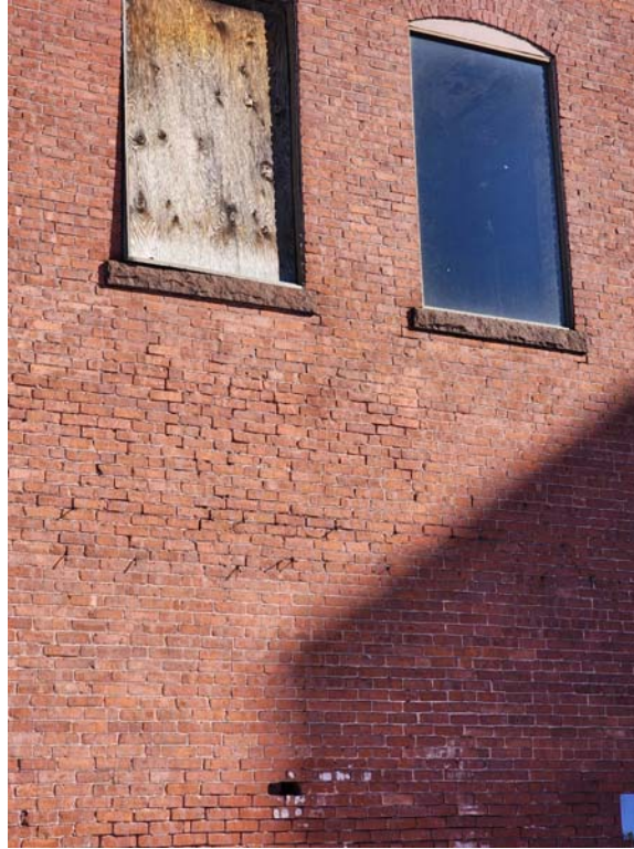
Photograph #36 – Exterior Masonry Joints
