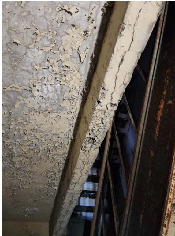
Photograph #17 – Cracked Concrete/Plaster Encasement
