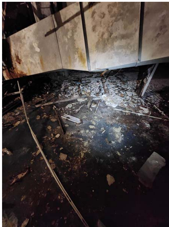
Photograph #5.1 – Ice on First Floor Slab
