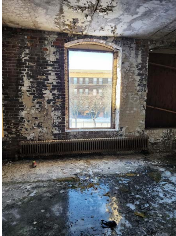
Photograph #1 – Ice on Upper Floor Level
