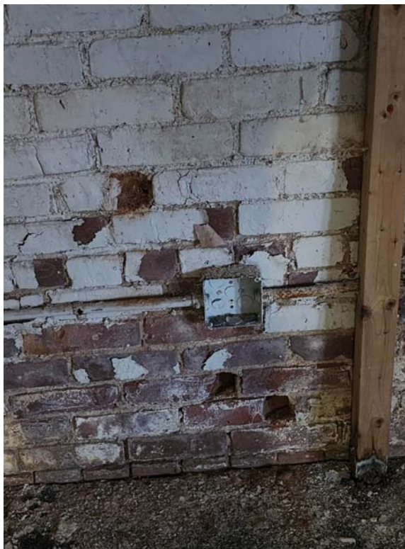
Photograph #29 – Deteriorated Interior Masonry
