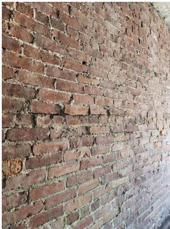
Photograph #31 – Deteriorated Interior Masonry
