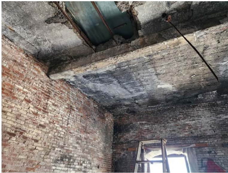
Photograph #15.1 – Cracked and Spalled Concrete Slab (Underside)
