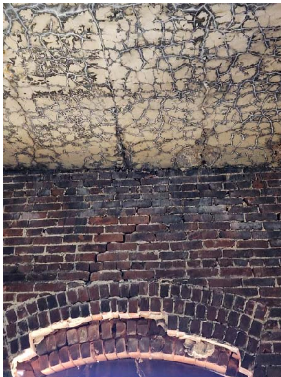
Photograph #33 – Cracked Interior Masonry
