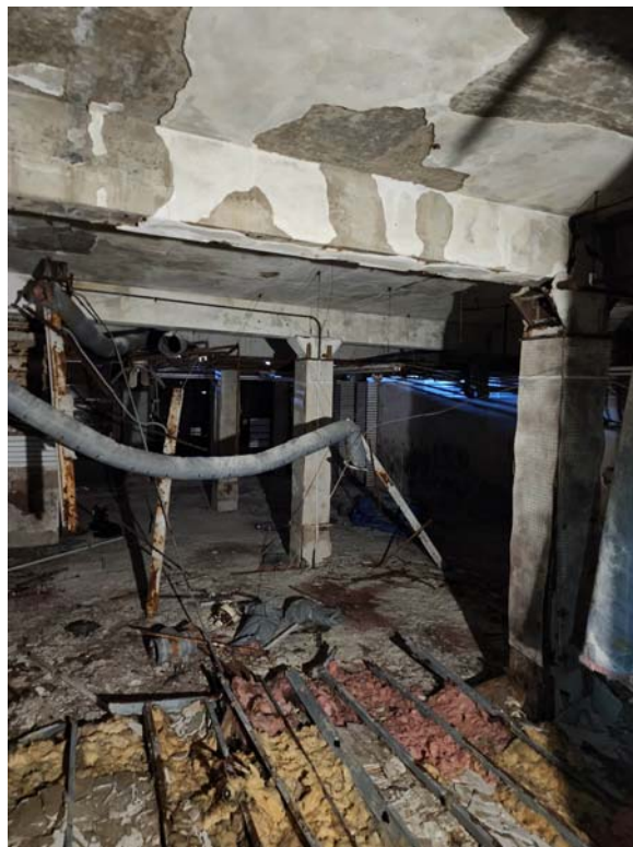
Photograph #27 – Corroded (Collapsed) Light-Gauge Metal Stud Wall
