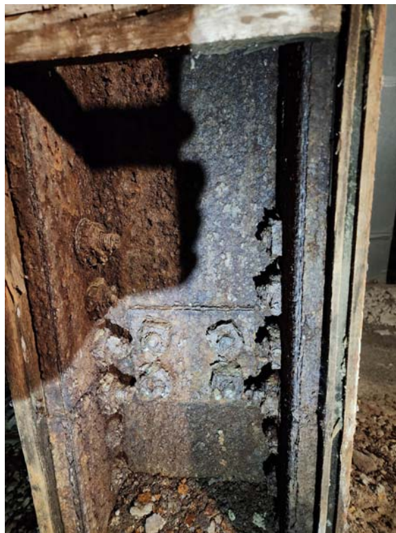
Photograph #21 – Corroded Steel Column
