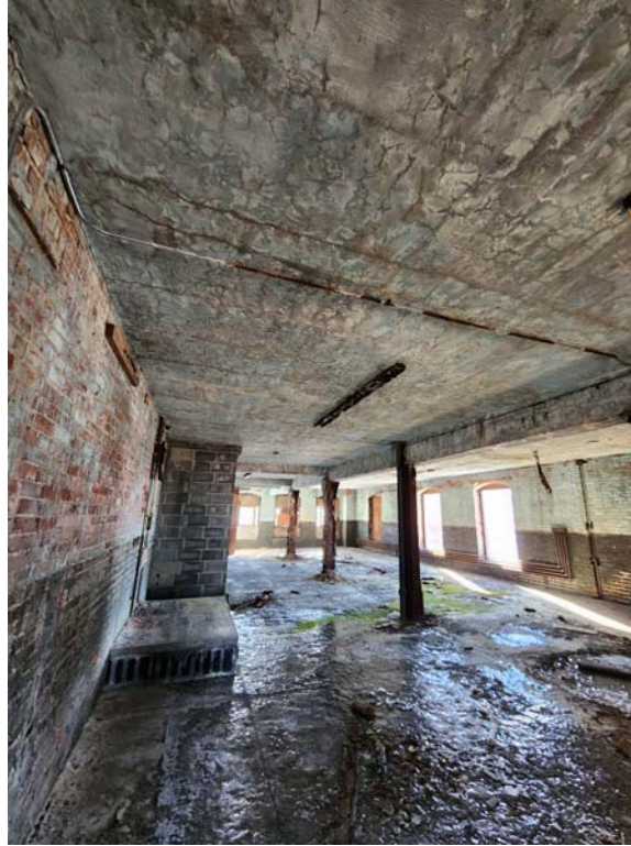
Photograph #5 – Ice on Upper Floor Level
