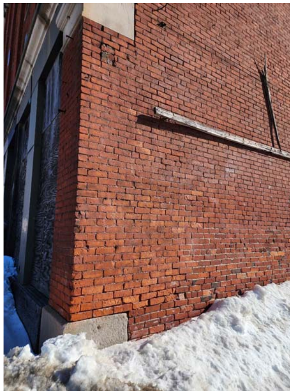
Photograph #37 – Exterior Masonry Joints
