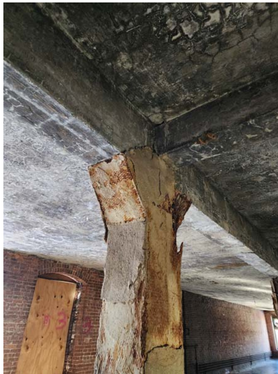
Photograph #25 – Rust Staining on Concrete/Plaster Encasement
