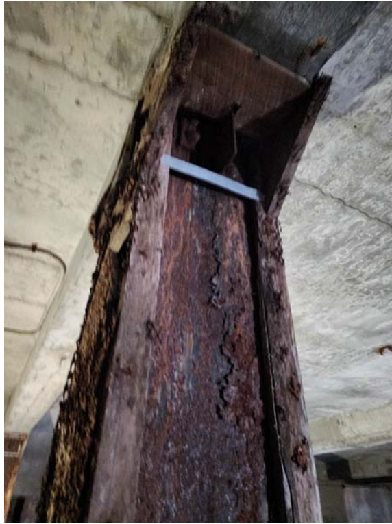
Photograph #22 – Corroded Steel Column
