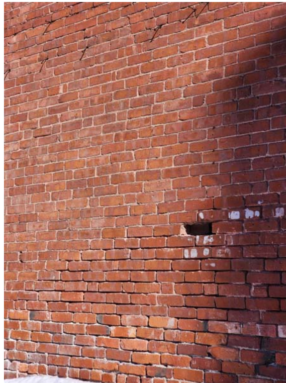
Photograph #35 – Exterior Masonry Joints
