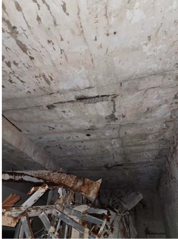
Photograph #26 – Corroded (Collapsed) Light-Gauge Metal Stud Wall
