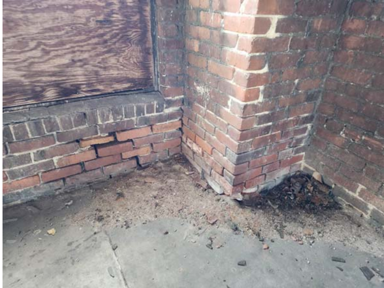
Photograph #34 – Deteriorated Interior Masonry
