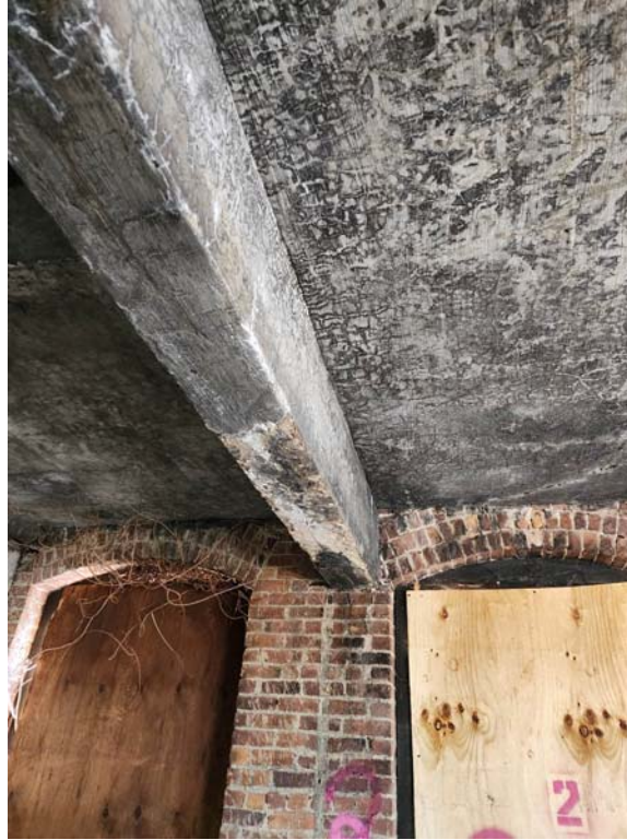
Photograph #20 – Cracked Concrete/Plaster Encasement
