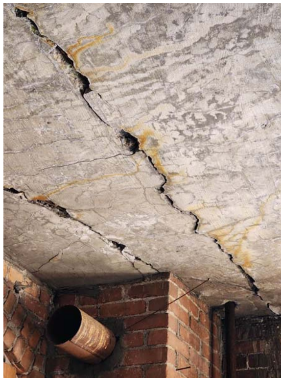
Photograph #14 – Cracked Concrete Slab (Underside)
