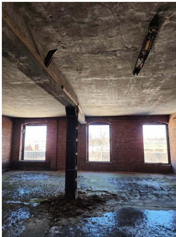
Photograph #4 – Ice on Upper Floor Level
