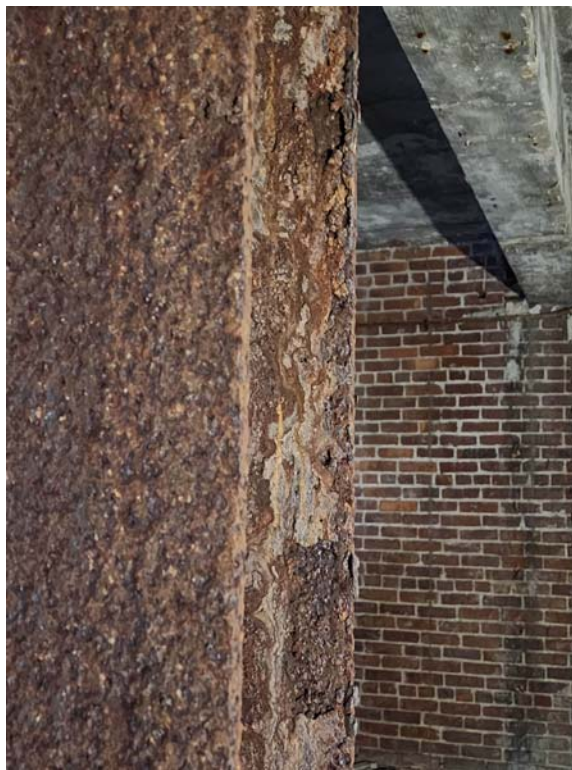
Photograph #23 – Corroded Steel Column
