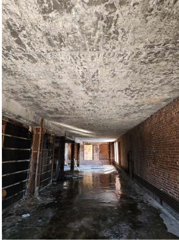
Photograph #3 – Ice on Upper Floor Level
