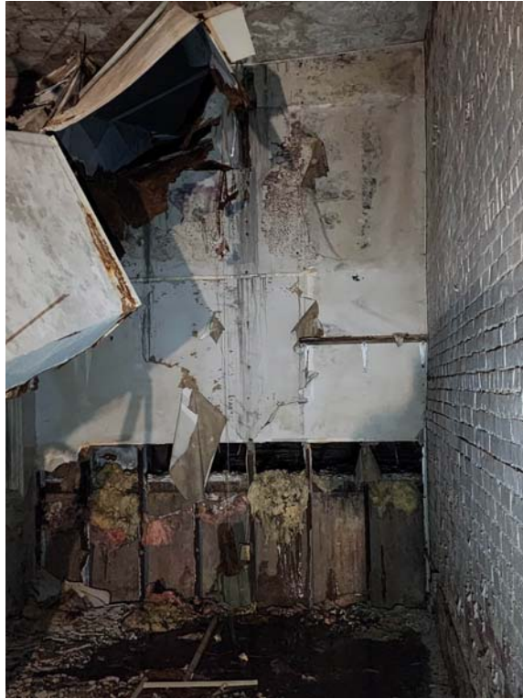
Photograph #28 – Corroded (Collapsed) Ductwork
