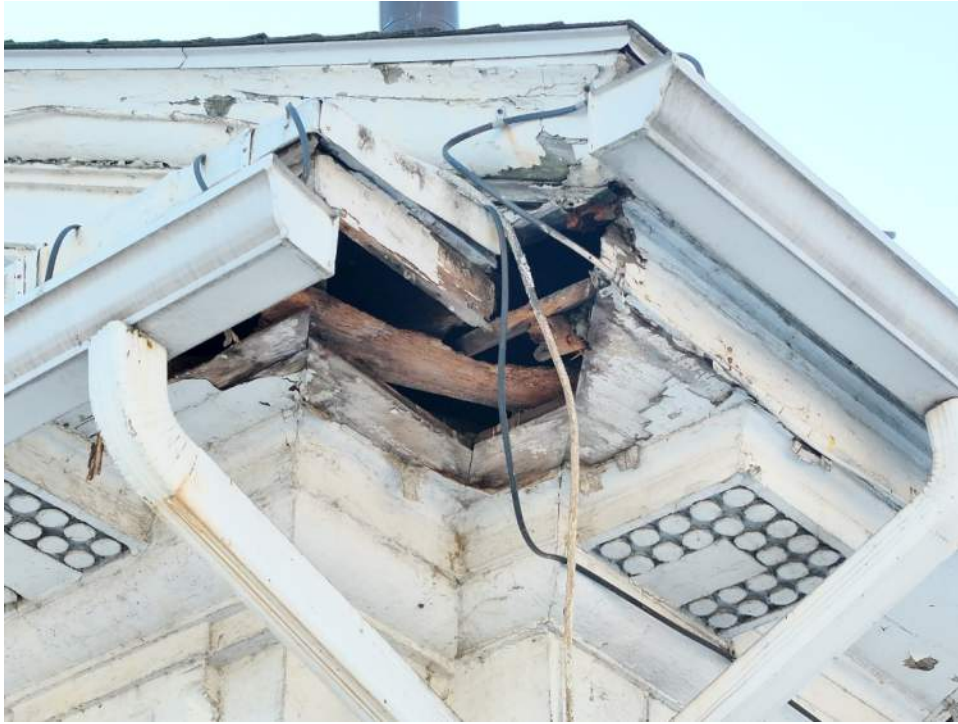
11. View of required repairs at the roof eave, rake, and soffit at the northeast corner of the Church.
