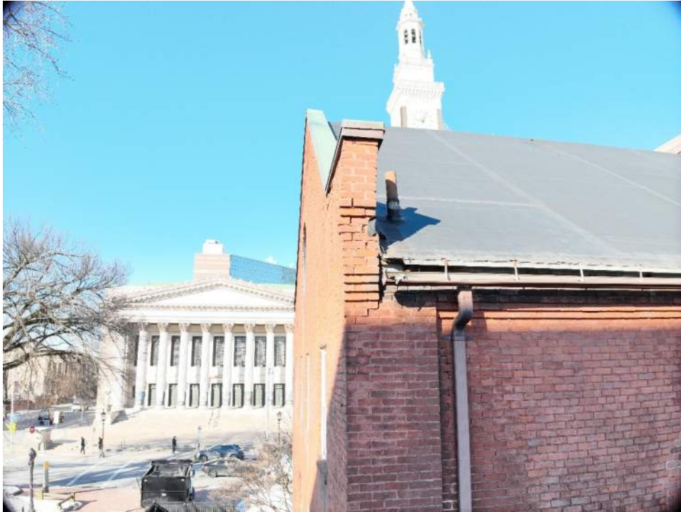
12. View of displaced masonry parapet at the southwest corner of the Parish House.
