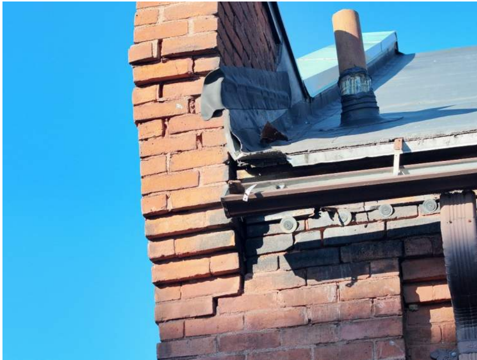
13. View of displaced masonry parapet at the southwest corner of the Parish House.
