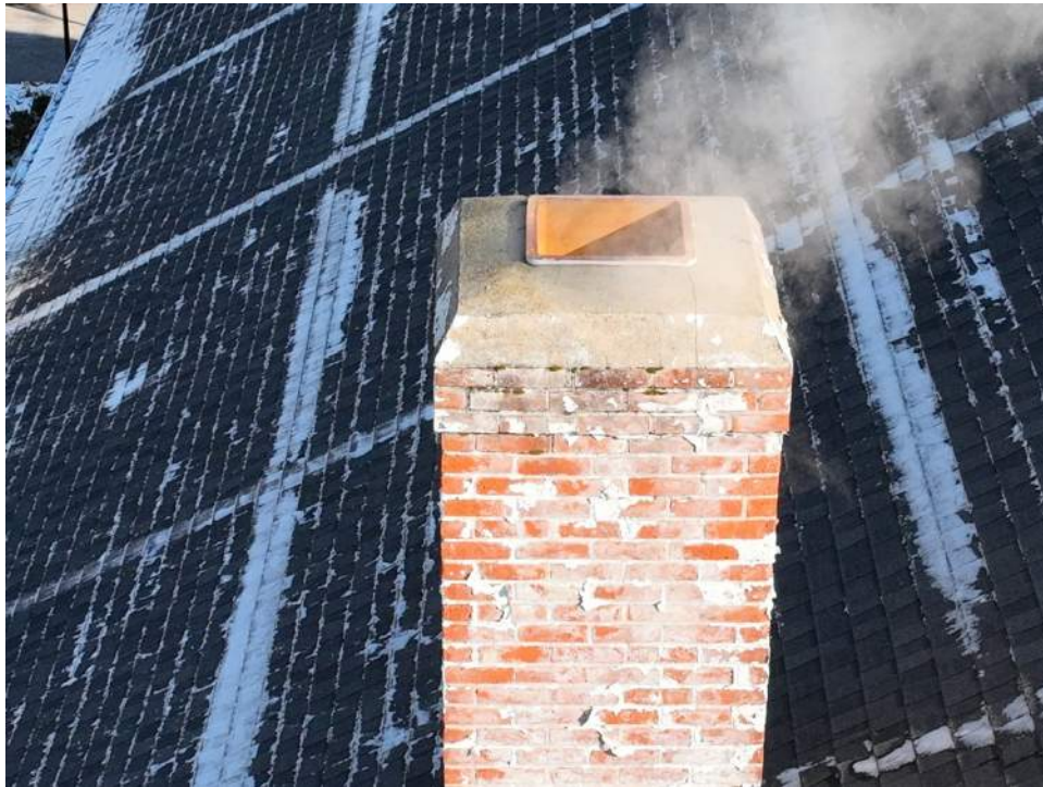
17. Church chimney scheduled for partial rebuild of upper courses, cap, and flue lining, and recoating.
