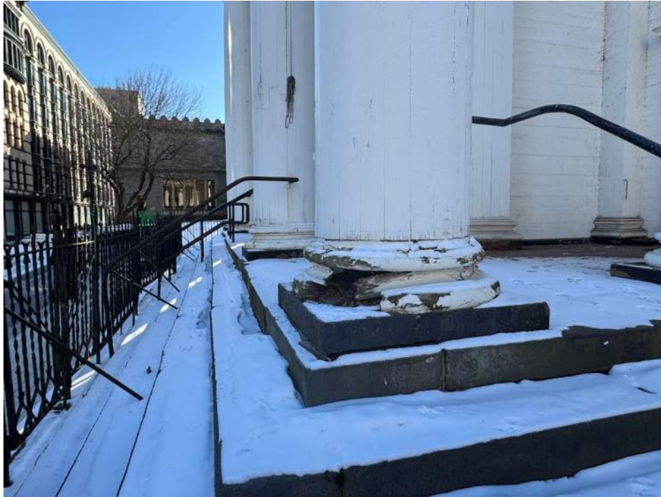
18. Typical Church wood column base scheduled for replacement.
