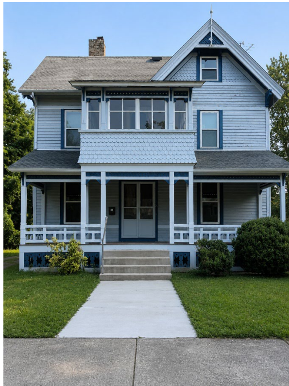
Current Siding Conditions
