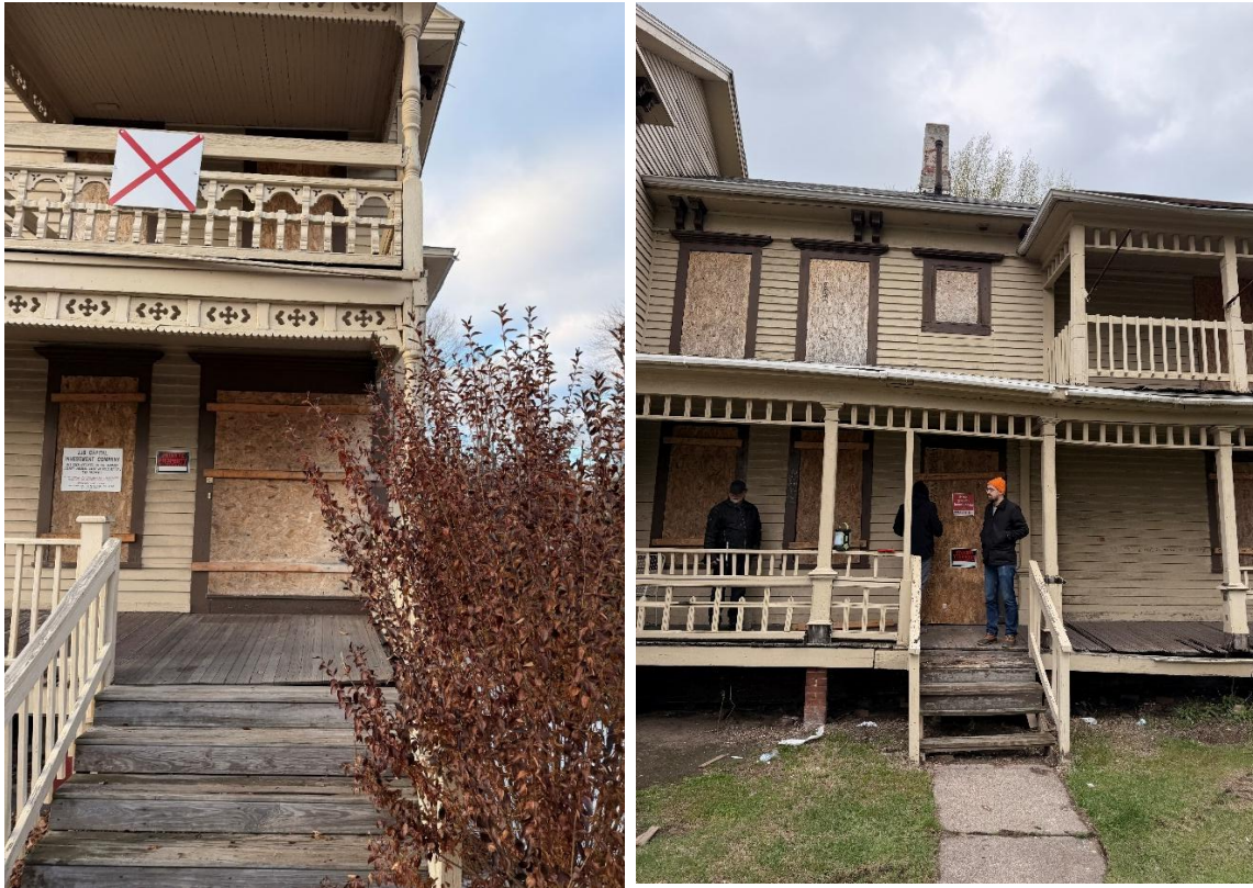
Fig. 14: Two Exterior Doors
