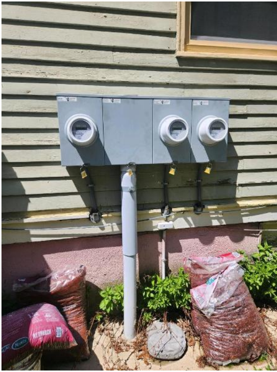
Electrical Evaluation / Meter Surroundings
