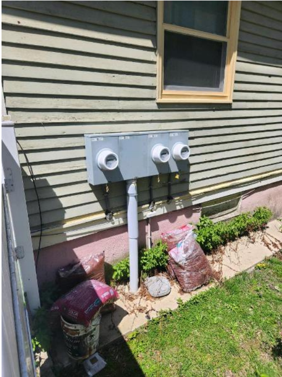
Electrical Evaluation / Meter Surroundings
