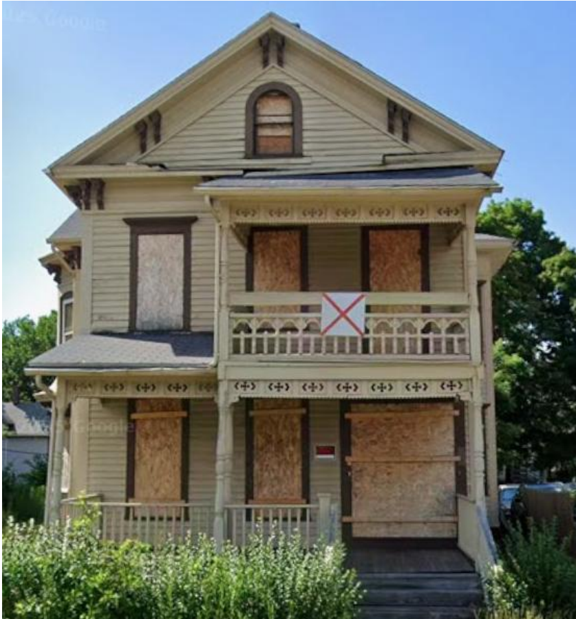
Fig.8: Exterior finishes Condition
