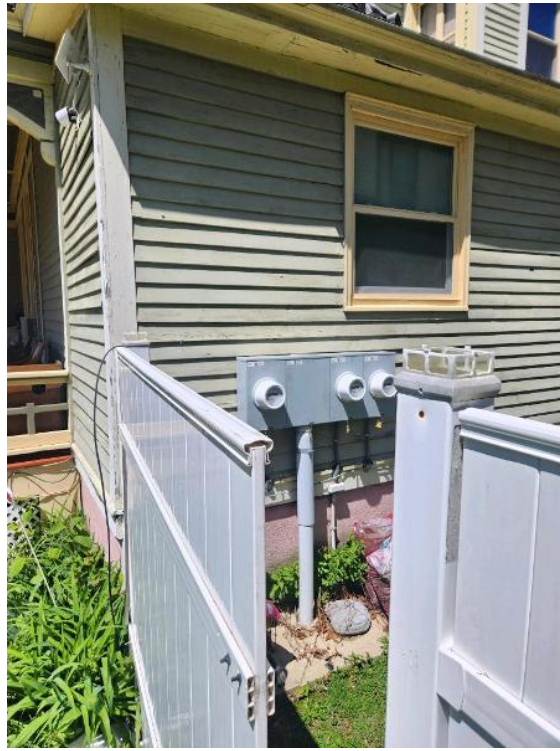
Electrical Evaluation / Meter Surroundings
