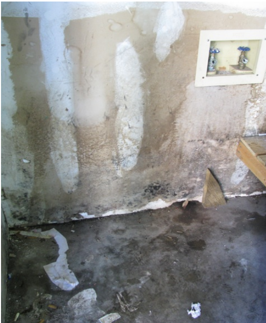
Mold on interior walls and floors.
