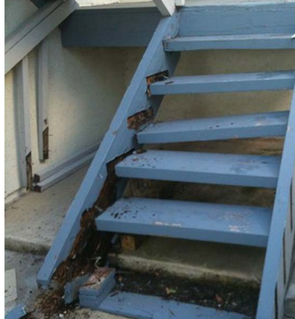
Rotting stairway missing treads, handrails, and guards.
