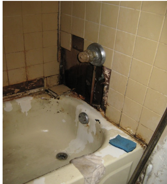
Missing tiles, rotting wall, mildew, and mold.
