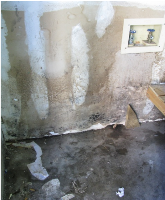
Mold on interior walls and floors.
