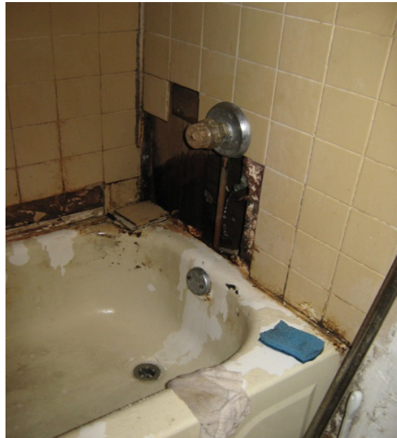
Missing tiles, rotting wall, mildew, and mold.
